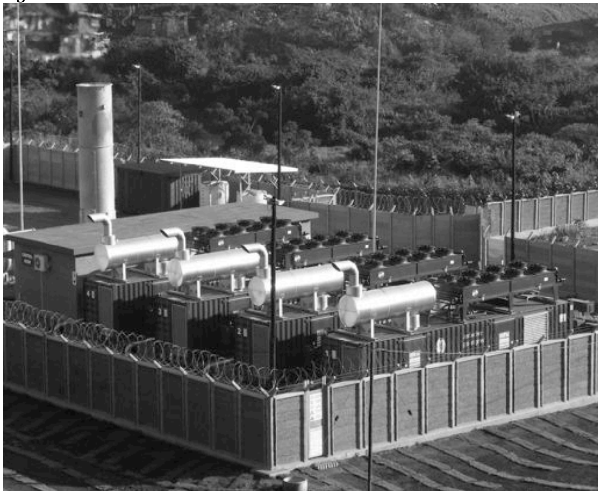
Figure 3.3: Bisasar Road CDM turbines
